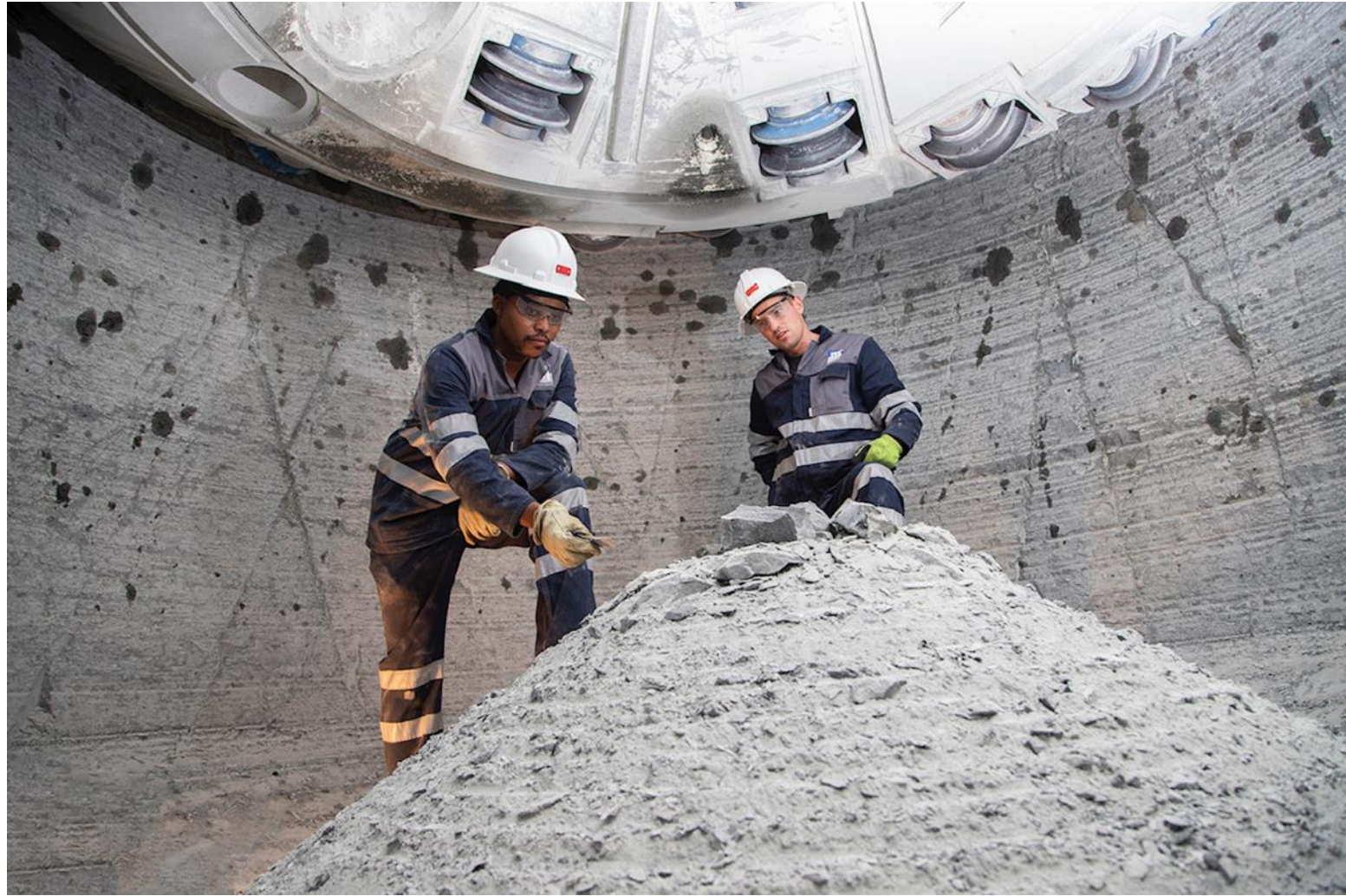
Image: Inspecting the shaft face during experimental testing, with the SBS cutterhead above
